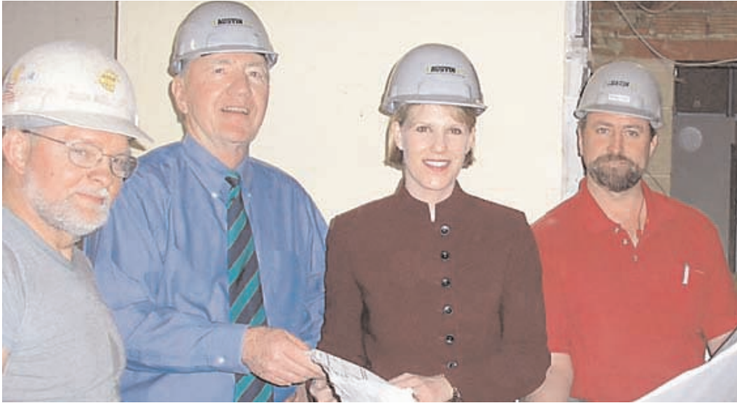
Dale Worden, E.E. Austin carpenter, looks over plans for a $600,000 renovation of the Robert H. Jackson Center with Rolland E. Kidder, Jackson Center executive director, state Sen. Cathy Young, and Brian Venn, E.E. Austin project supervisor.
